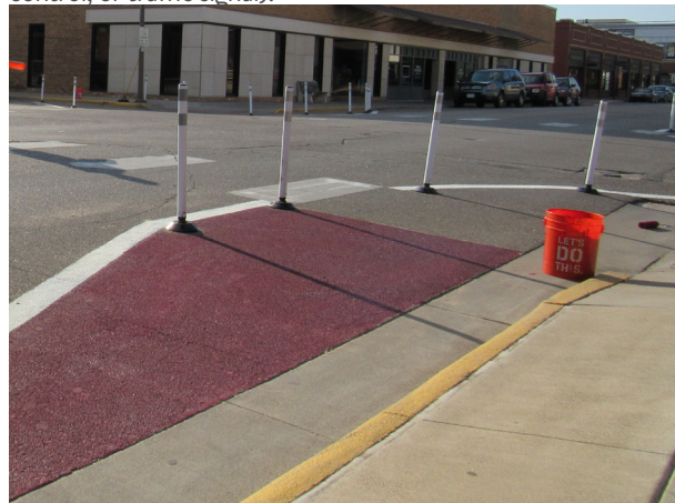
Image 5.04: Rust colored paint in a curb extension outlined with white paint
