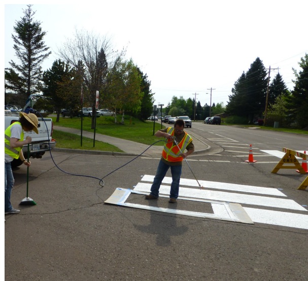
Image 4.04: Demonstration team installing crosswalk markings. Paint may be applied with a sprayer (as pictured) or a roller.
